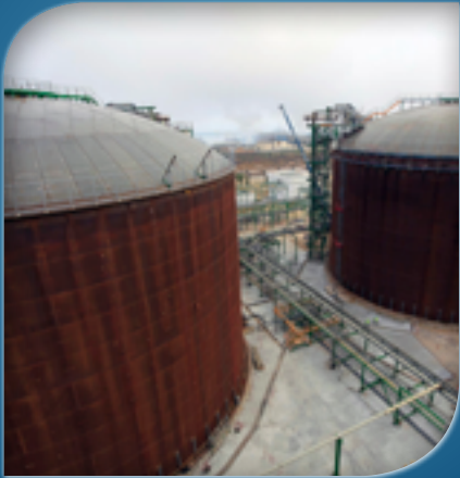
AMMONIA STORAGE AND DISTRIBUTION UNIT
