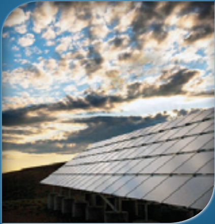
ASKANDRA CONCENTRATED SOLAR POWER PLANT
